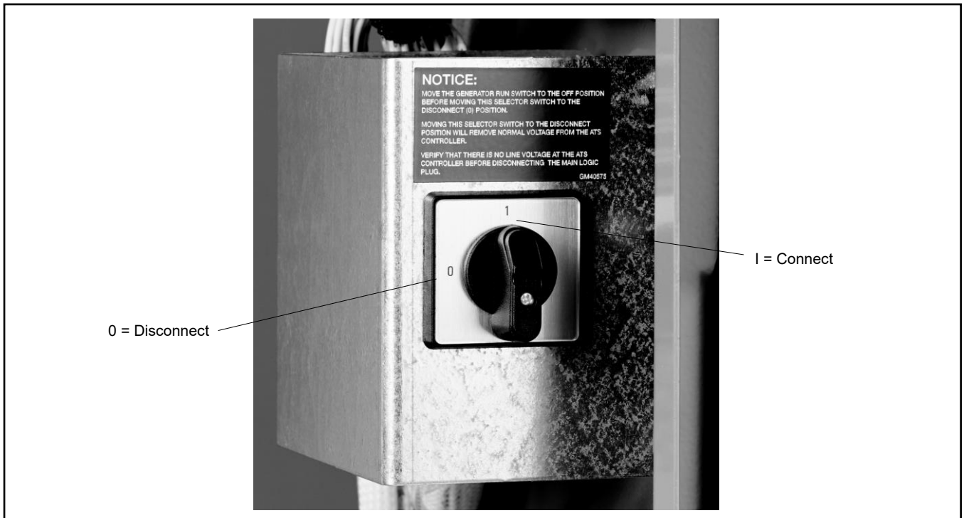
Figure 69 Controller Disconnect Switch
