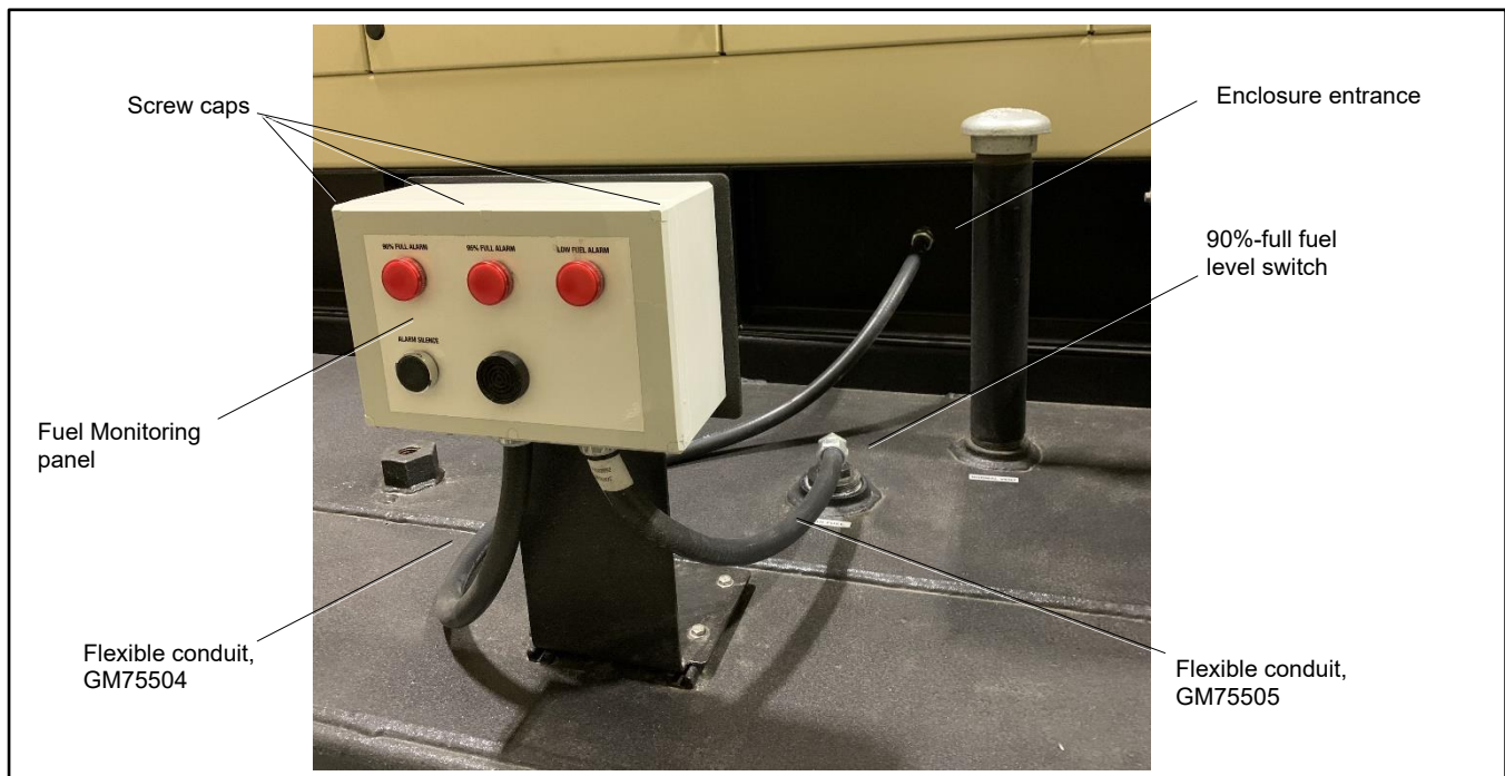
Figure 50 Fuel Monitoring Panel, Overview
