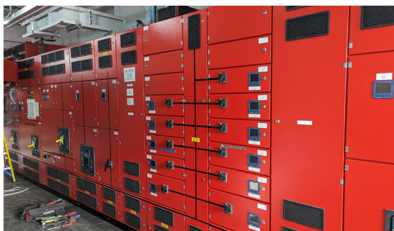
Figure 4 Containerized N+1 UPS system
