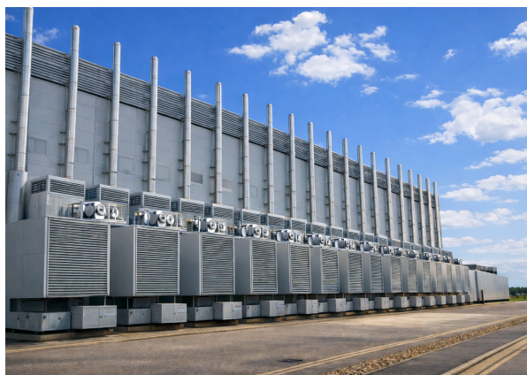
Figure 2 Standby Generators at a Hyperscale Data Center
